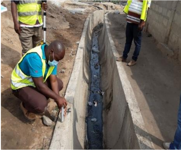
Picture 3: Measuring the concrete strength of a drain (using the Schmidt hammer).
