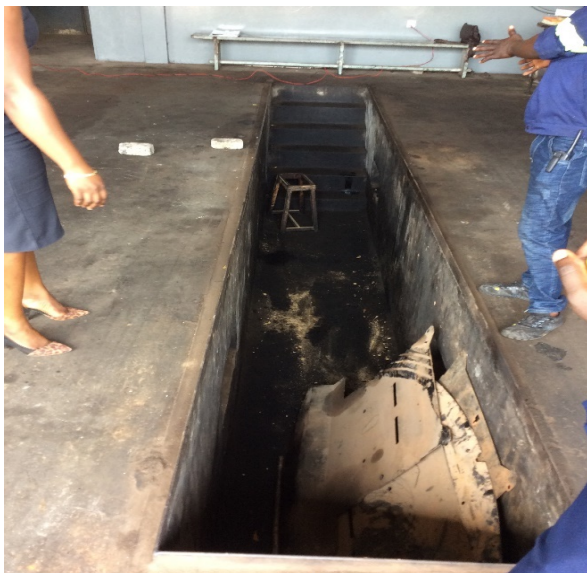
Picture 1: Audit team's inspection of servicing pit at NAS workshop in Accra
